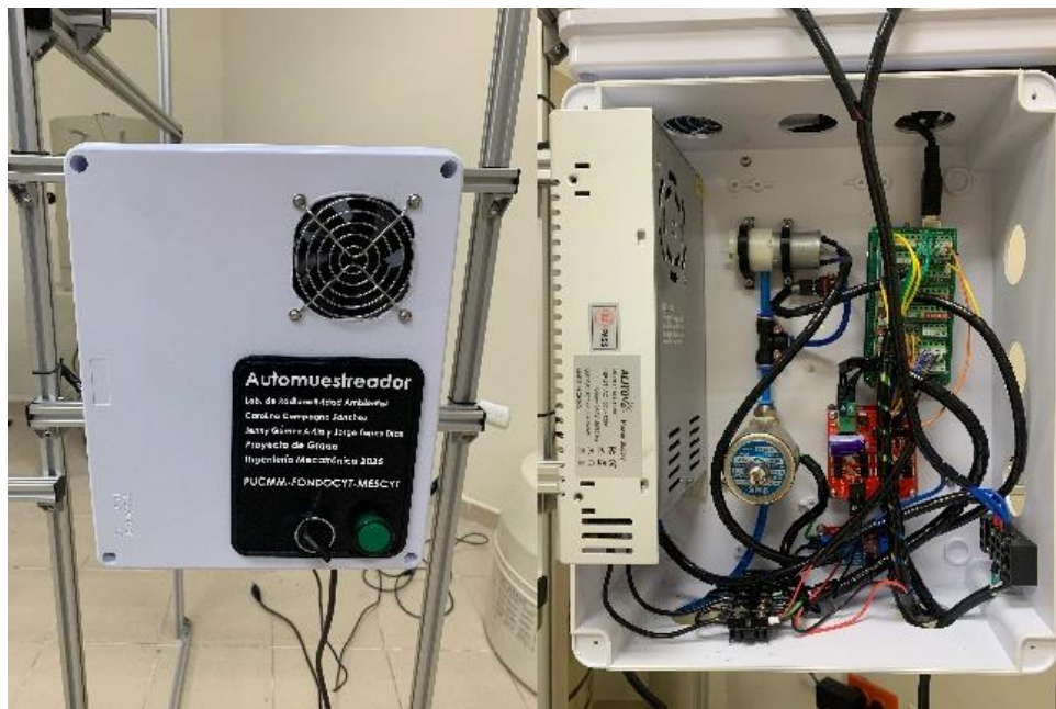
Figure 8: Exterior (cover) and interior of the autosampler's electrical panel
